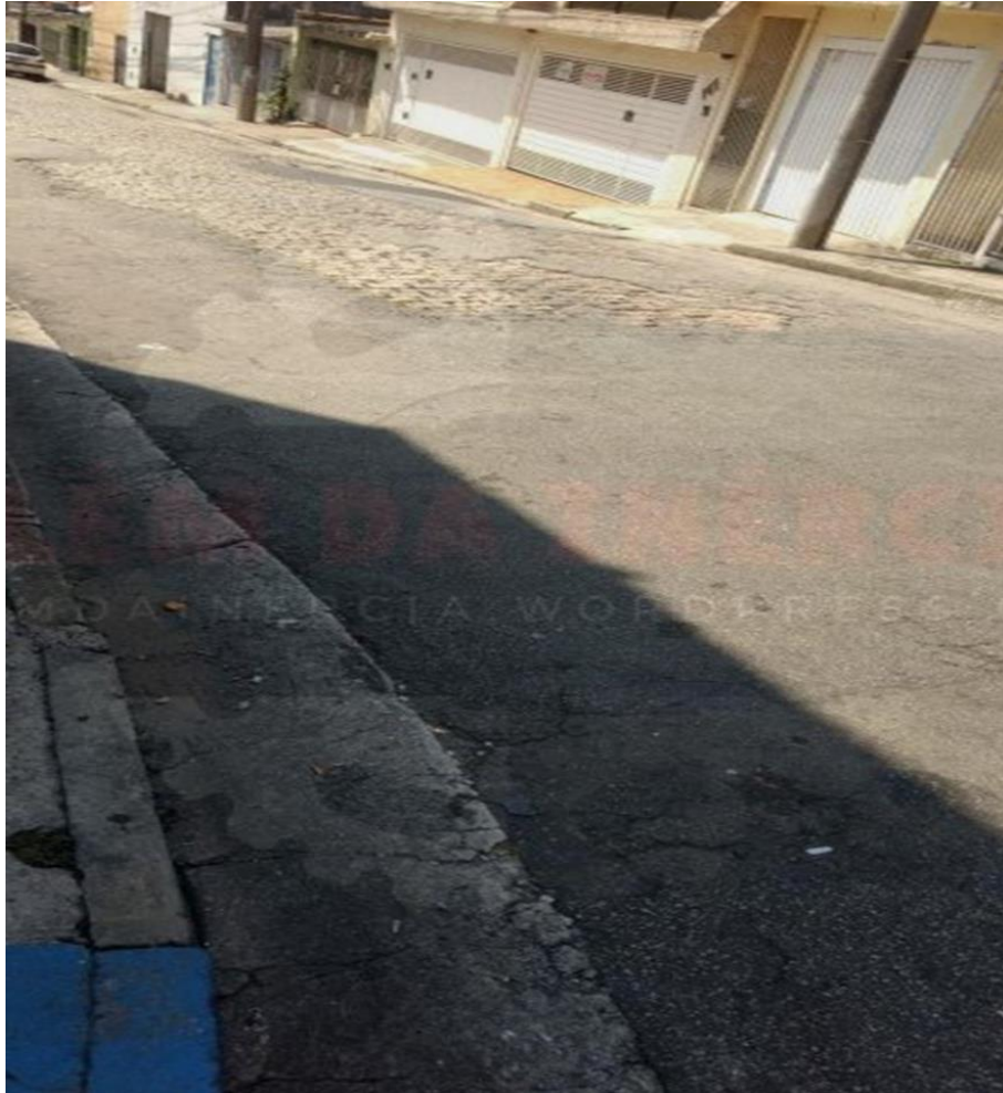
Figure 14 - Lack of adhesion on cobblestones. Source: Author (2018)
