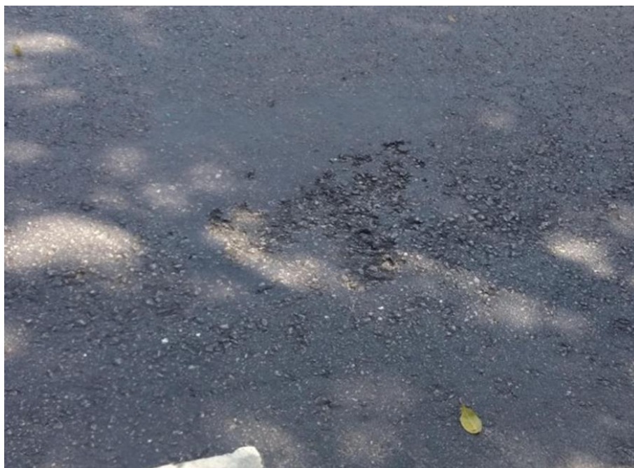
Figure 17 - Bleeding. Source: Author (2018)
