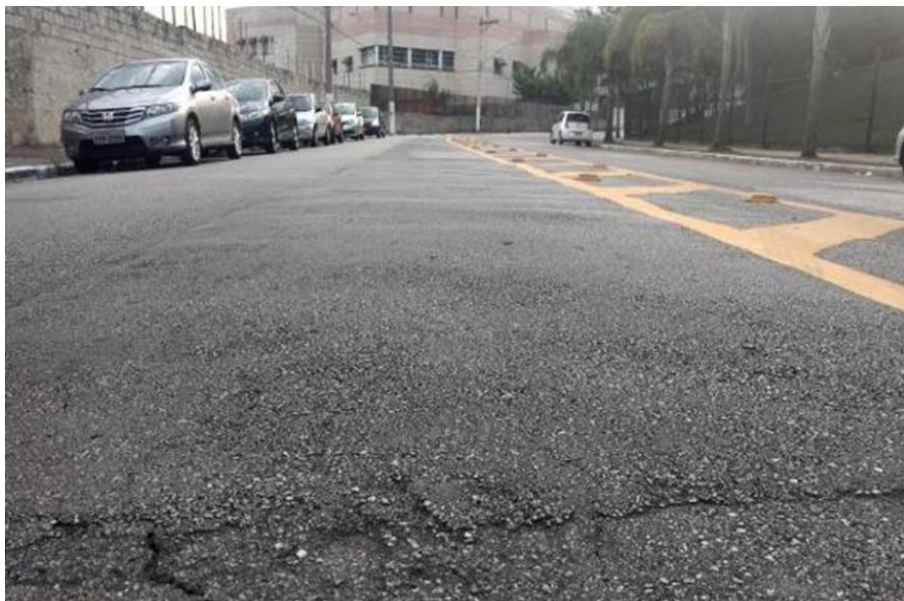
Figure 11 - Shoving and Corrugation. Source: Author (2018)
