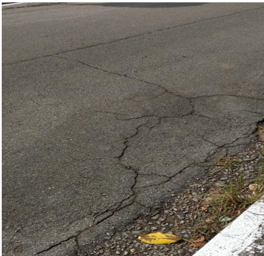
Figure 18 - Edge Cracking. Source: Author (2018)
