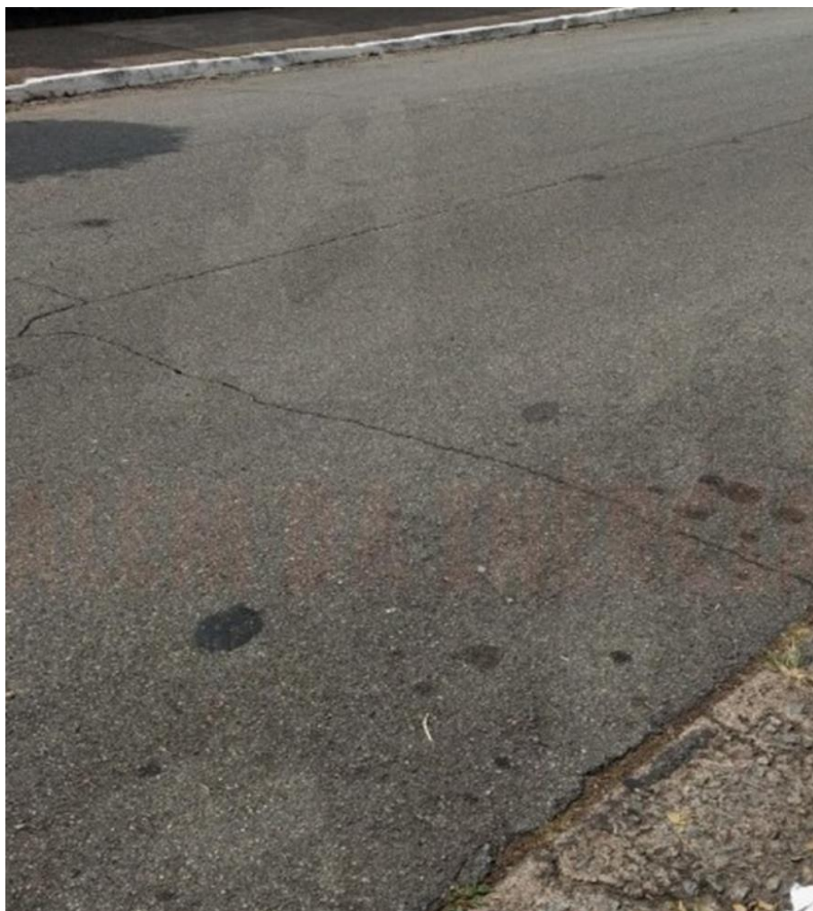
Figure 15 - Transverse Cracking. Source: Author (2018)
