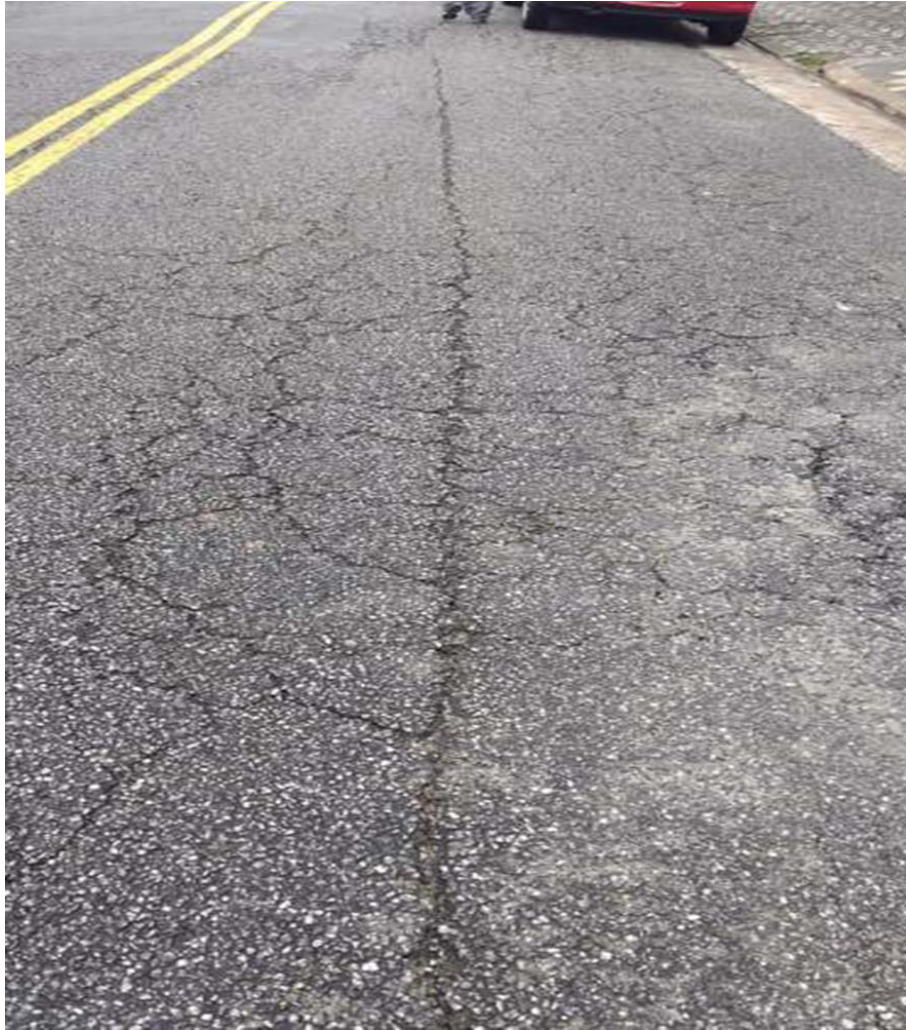
Figure 8 - Longitudinal Cracking. Source: Author (2017)
