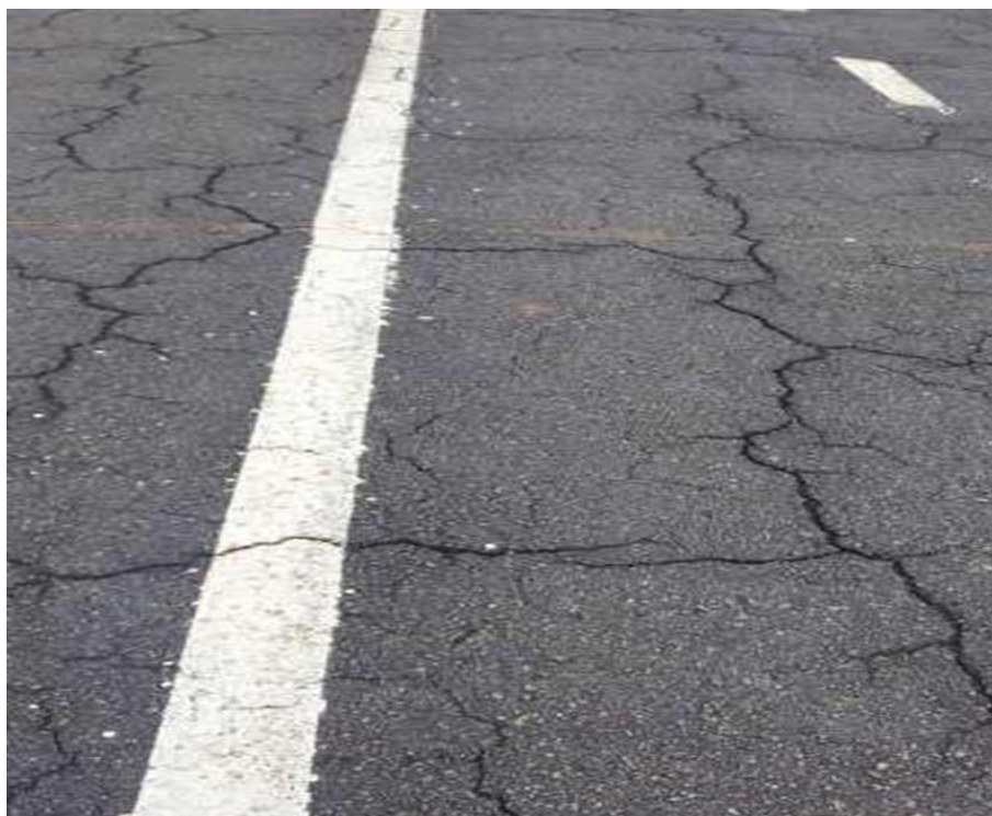
Figure 7 - Block cracking. Source: Author (2018)
