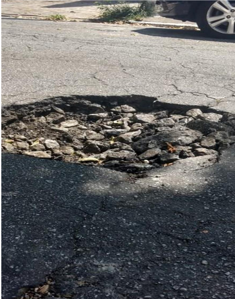
Figure 9 - Potholes. Source: Author (2018)
