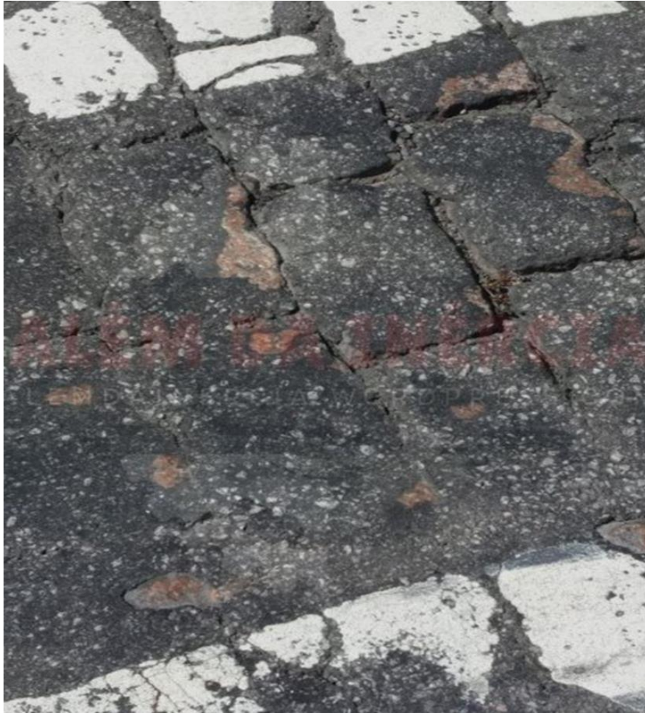
Figure 13 - Reflection Cracking. Source: Author (2018)
