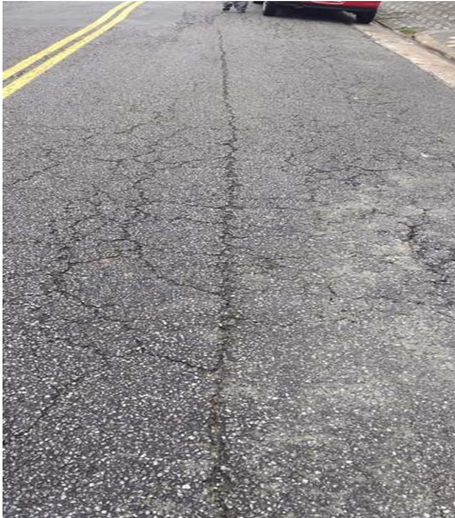
Figure 8 - Longitudinal Cracking. Source: Author (2017)
