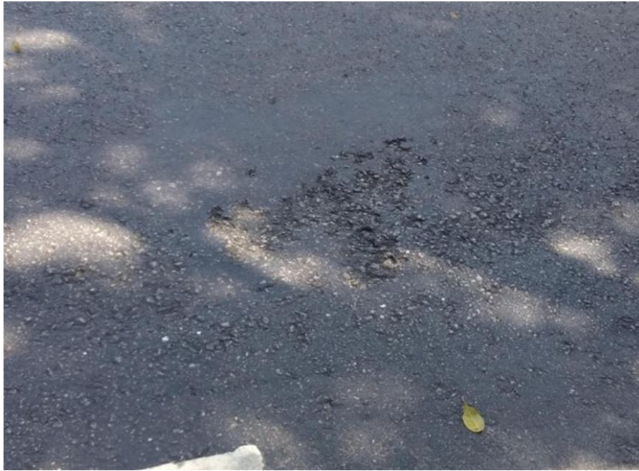
Figure 17 - Bleeding. Source: Author (2018)
