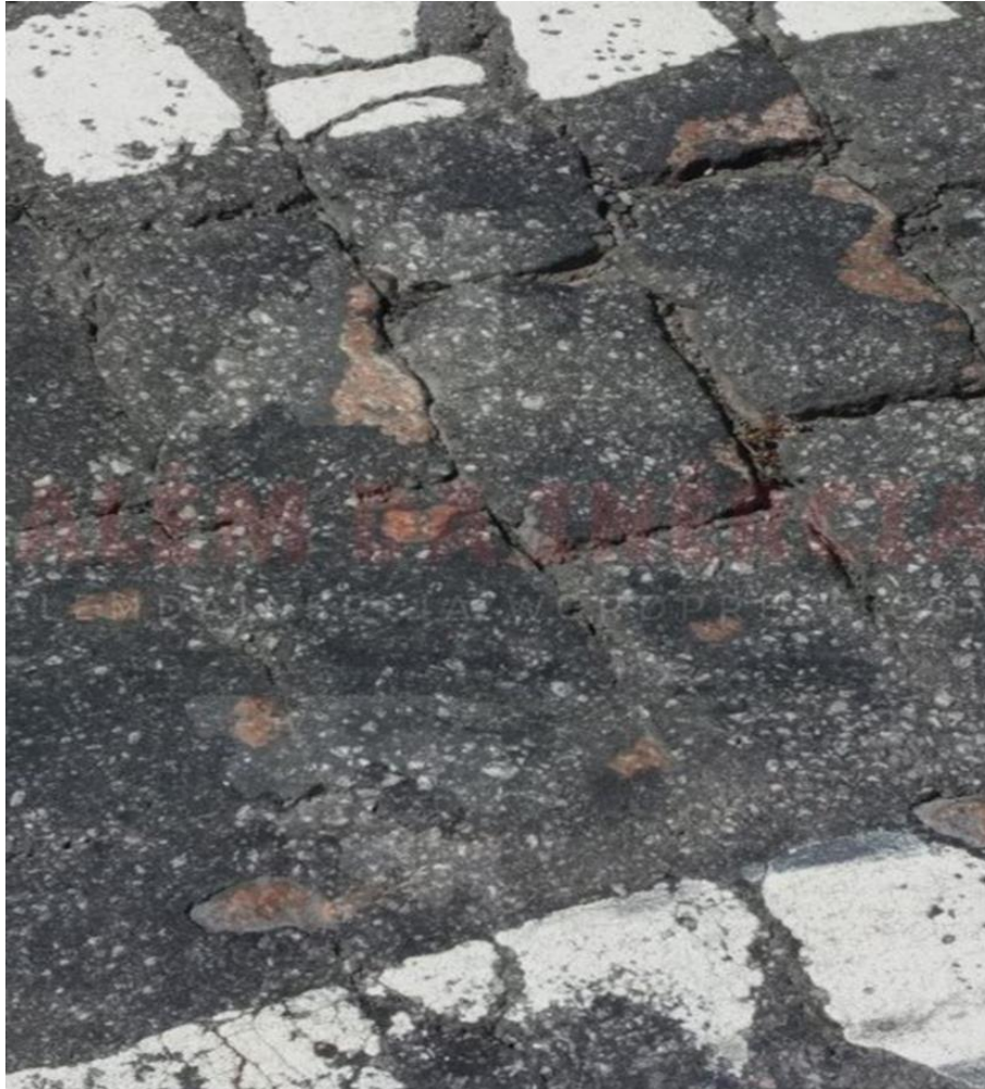
Figure 13 - Reflection Cracking. Source: Author (2018)
