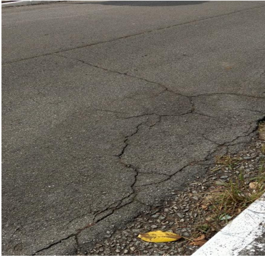
Figure 18 - Edge Cracking. Source: Author (2018)
