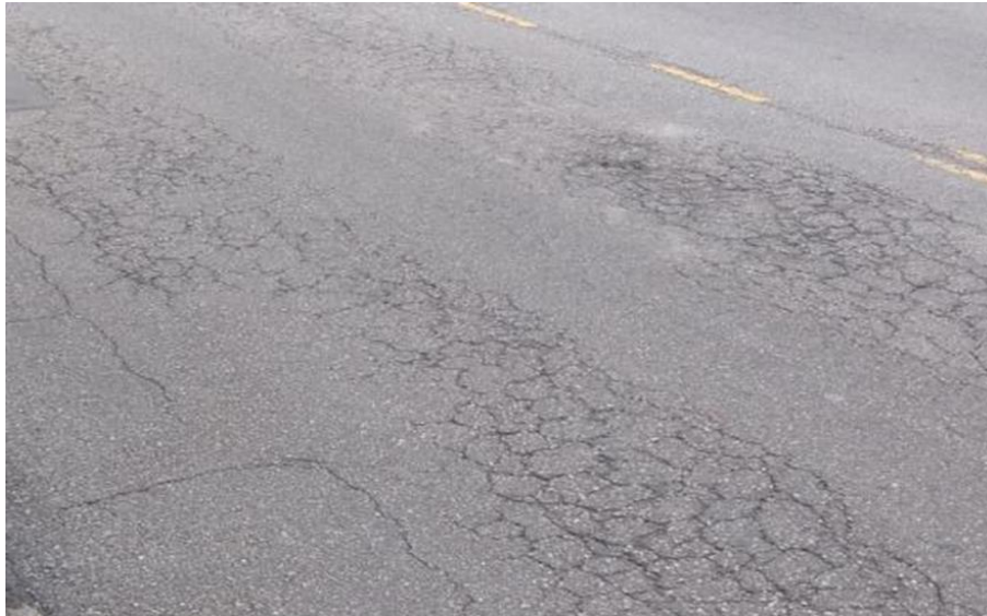
Figure 6 - Permanent Deformation (Rutting) and Fatigue Cracking in the wheel track.
