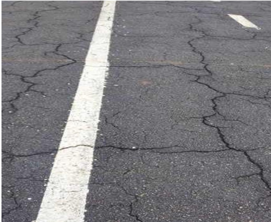
Figure 7 - Block cracking. Source: Author (2018)
