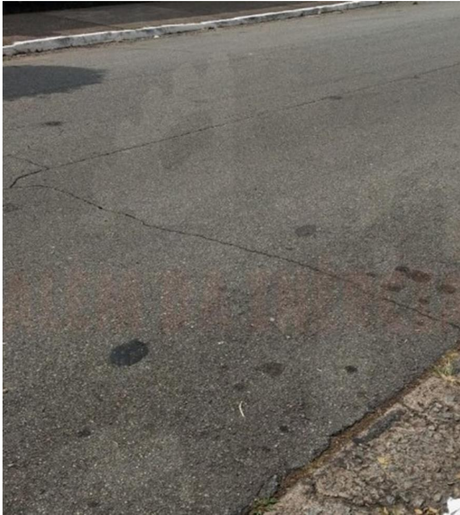
Figure 15 - Transverse Cracking. Source: Author (2018)
