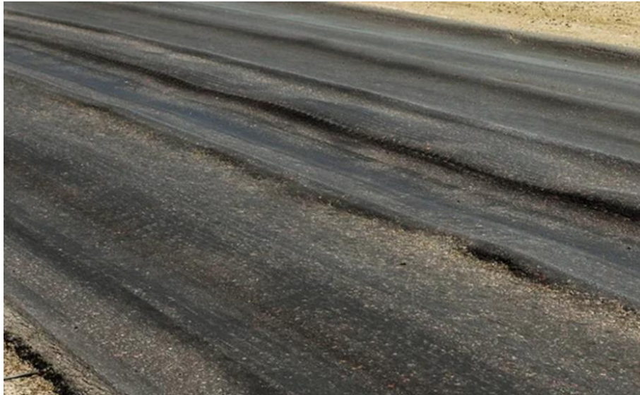
Figure 20 - Deformations or ripples caused by the passage of very heavy vehicles and/or poor quality of the applied base
